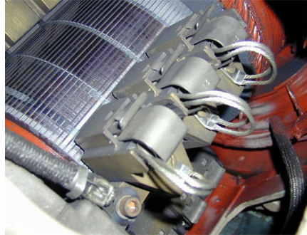
Figure 2: Heavy contamination attacking copper
